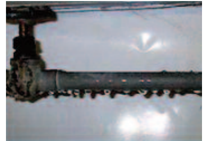
Moisture condensing on the outside of compressed air pipework (sweating)
