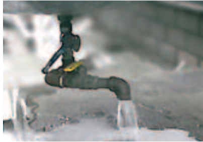
Untreated compressed air does not prevent large amounts of water from collecting in air receivers and downstream piping.
